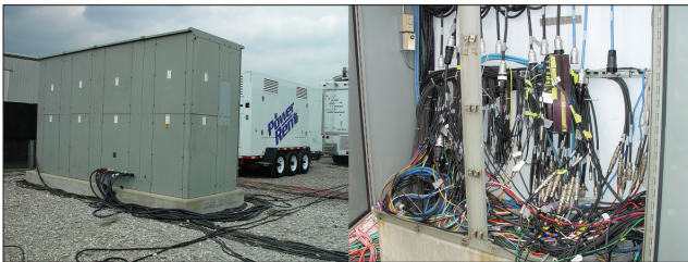
Figure 7.23 Power transformer for IMS and ESPN side of the compound could provide 1MW of power. The ABC side of the compound had 1.25MW available. Right is one of the I/O panels into the compound near the IMS trucks, where some of the 33 cameras and 58 mics hit the compound.
